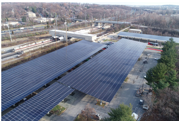
Pictured: Solar carports at Cheverly Metrorail Station
