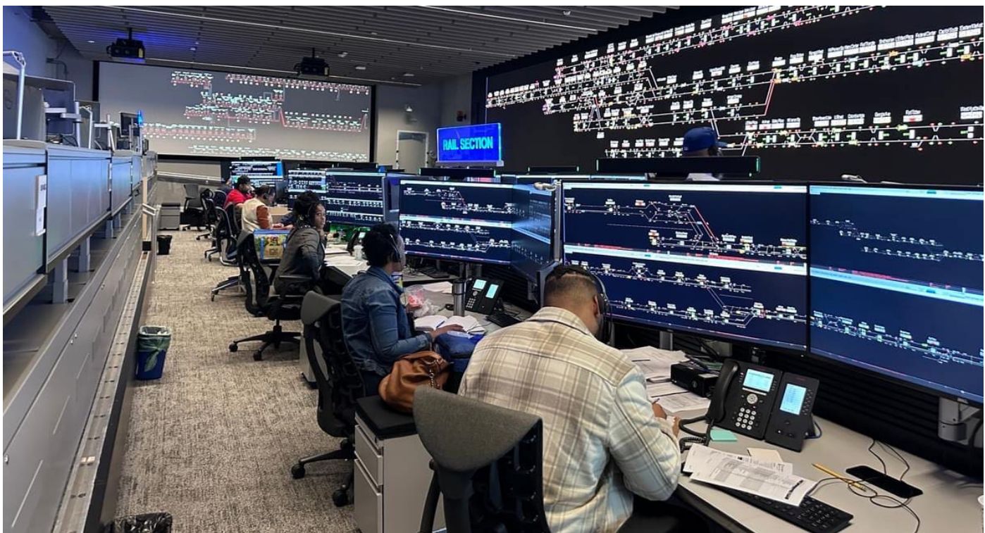
Pictured: Metro Integrated Command and Communications Center
