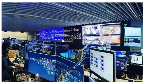
Metro Integrated Command & Communications Center (MICC)
