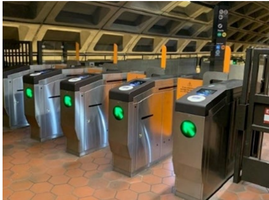
Example: Upgraded faregates at L'Enfant Plaza
