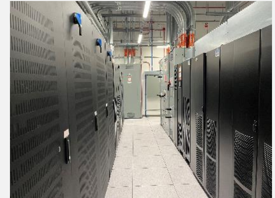
IT Infrastructure at Eisenhower Ave Office
